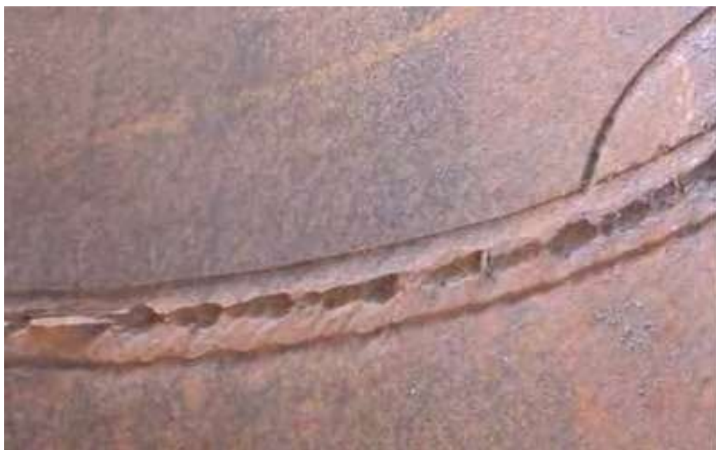
Figure 3-2-3—Preferential weld corrosion in lean amine. (Reference 5)
