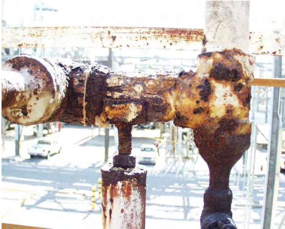
Figure 3-22-8—CUI of a carbon steel level bridge.
