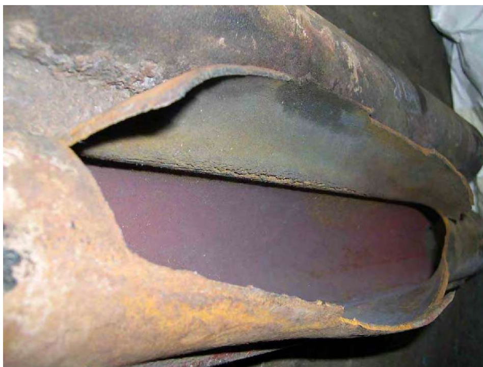
Figure 3-21-1—Corrosion fatigue failure of a boiler tube.
