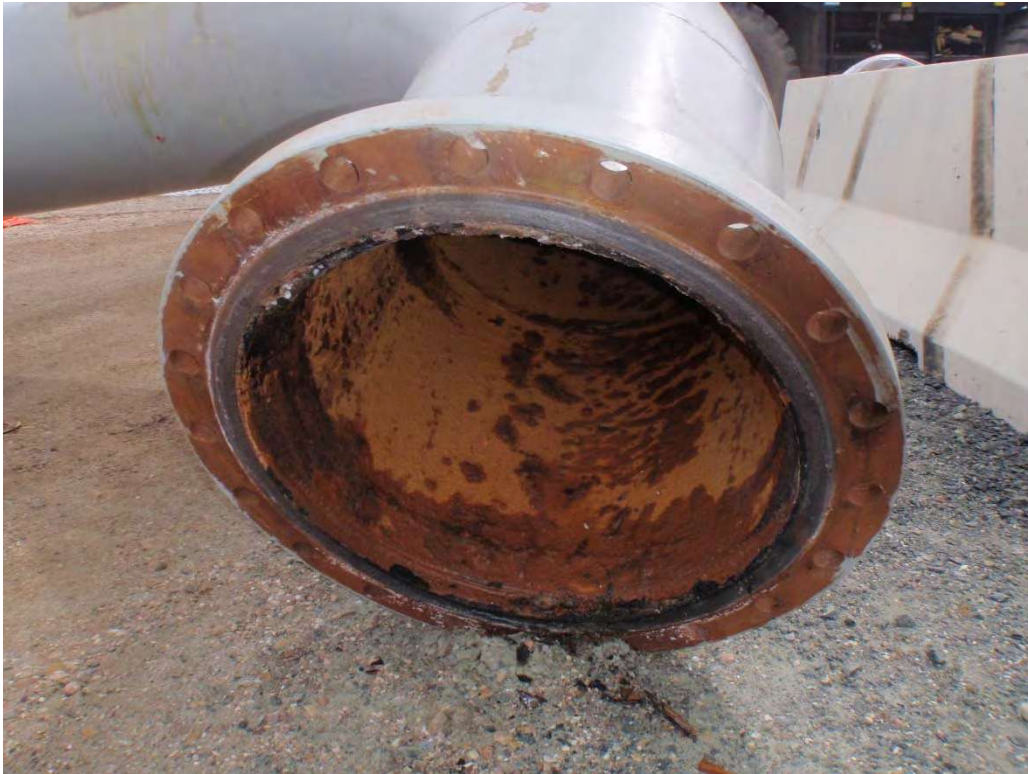
Figure 3-10-1 – Brine corrosion at a flange connection.
