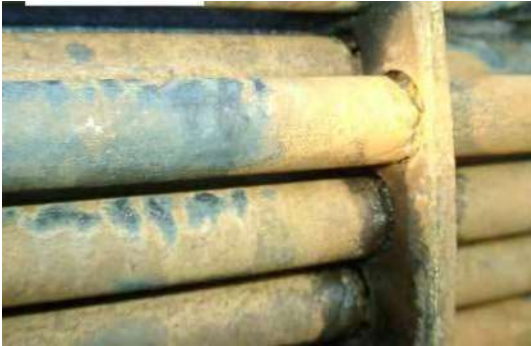
Figure 3-62-2—Accelerated sulfuric acid corrosion under a baffle.
