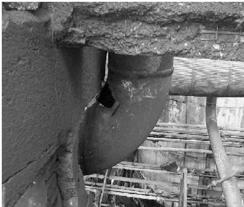
Figure 3-61-7—Sulfidation failure of piping elbow.
