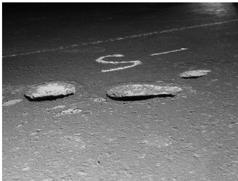
Figure 3-45-1—MIC on a diesel tank bottom.
