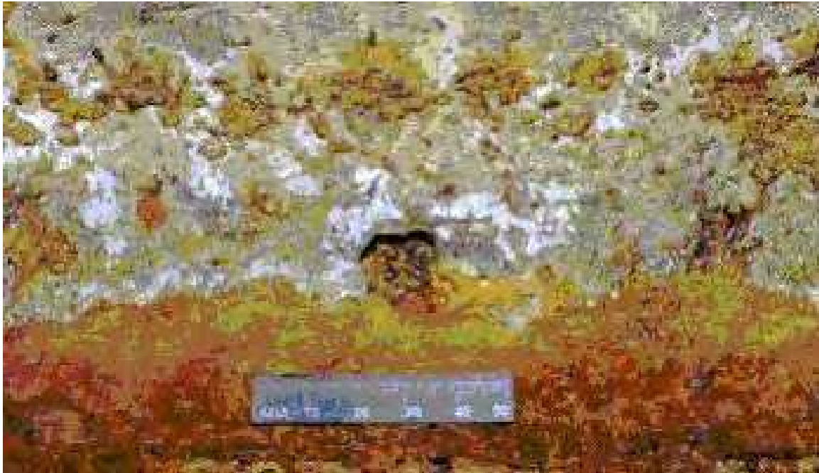
Figure 3-45-4—Oil line with MIC damage beneath tubercles.
